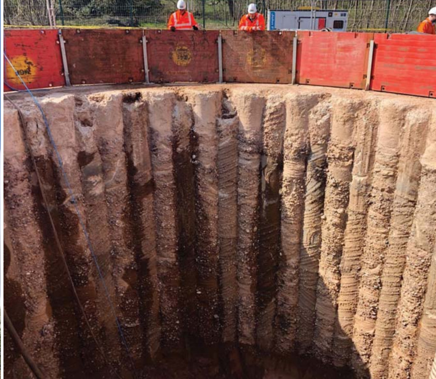
Above: HP11 secant piled reception shaft excavated to formation level, immediately after excavation, April 2020.
